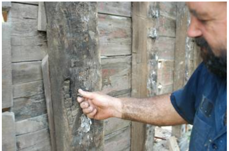
Edward pulls a charred cinder from the north chimney stud on the east wall, 8/29.
